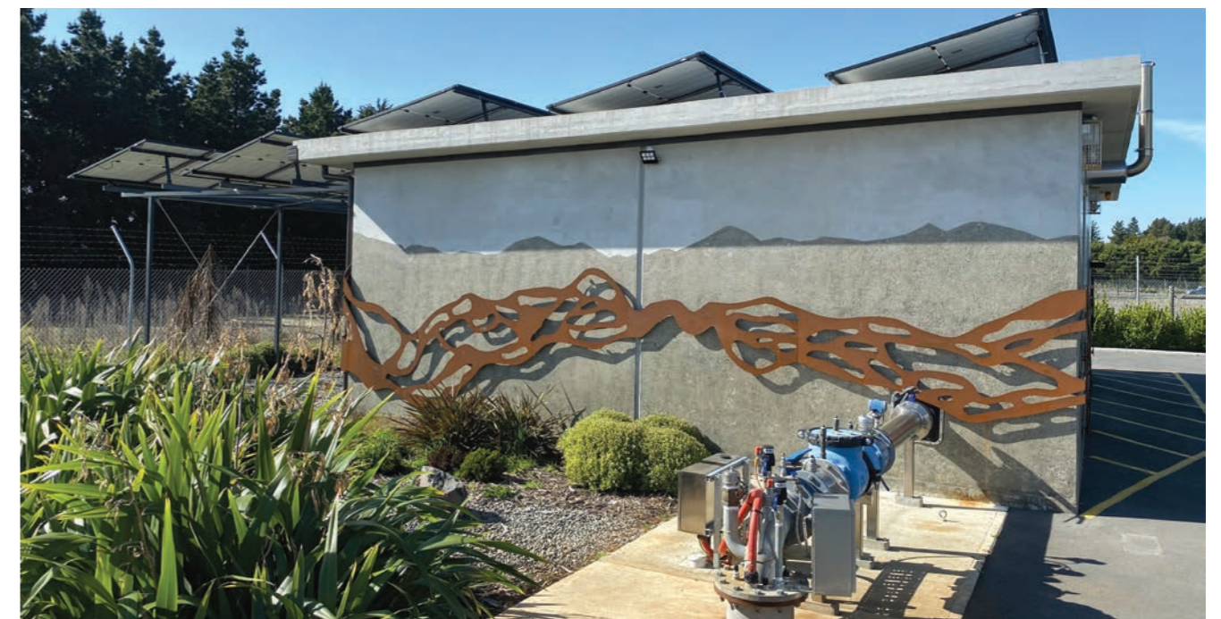
Our first solar panels have been installed at this potable water treatment plant to reduce carbon emissions and operating costs while providing safe and compliant water across the campus.
